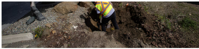
Workers dig a trench which will allow them to install underground infrastructure at Hidden Trails, a Homex development in Kamloops.
