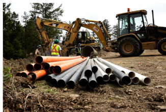
Labourers work to install underground infrastructure on undeveloped land at Hidden Trails.
